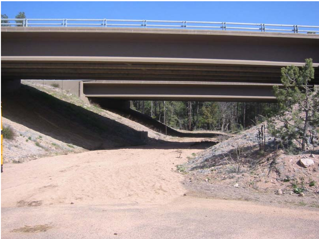
A recently built underpass designed to assist elk in moving back and forth between a riparian area at night and a pine forest in the day. Note the gentle slopes along the side of the structure and open line of sight.
